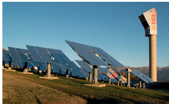
CNRS PROMES Central Tower thermodynamic solar power plant
