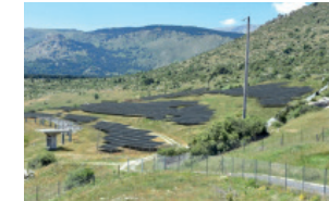
Engie Green Bifacial photovoltaic solar power plant
