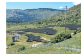
Engie Green Central fotovoltaica bifacial
